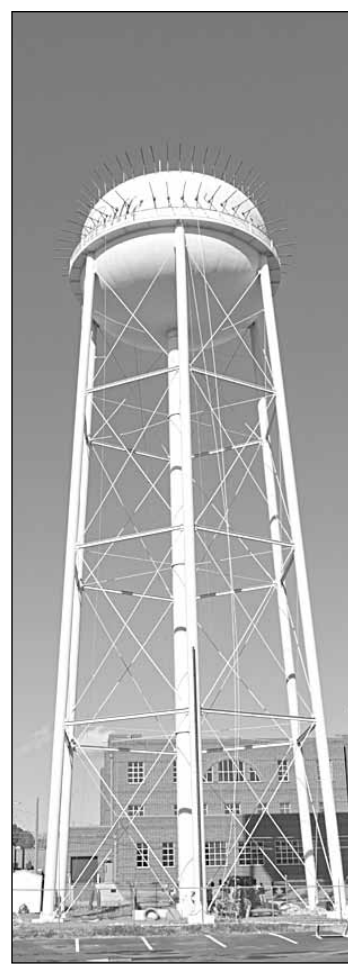
A $82,313 contract is providing the repainting, repairs and removal of lead-based paint from the 1950s era Smith Street water tower.
