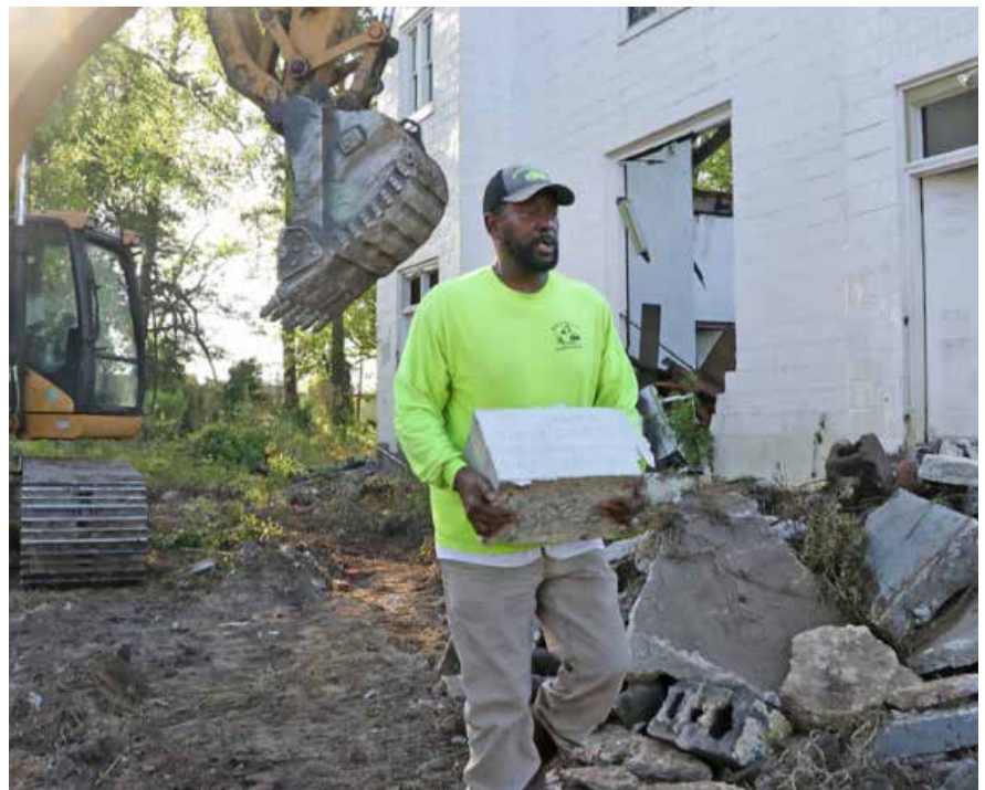
From a recent article in The News Reporter, this photo shows Darryl McNeill of Morgan Trucking carrying the cornerstone away from St. James A.M.E. Church in Whiteville before a crew demolished the sanctuary. After buying the church property, DOT allowed the congregation to remove the stained glass windows and cornerstone. The church plans to display them at its new sanctuary on Williamson Street.
