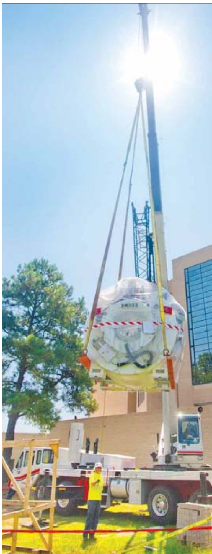
In August, workers use a crane to move Columbus Regional Healthcare's new 11,000-pound MRI magnet from a flatbed to its new home in the hospital's imaging department. The MRI opened in September.
