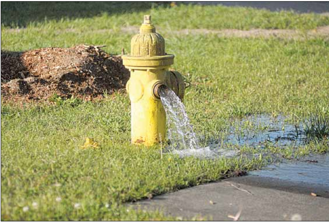
Hydrants are running throughout Whiteville to help avoid pressure problems while the city renovates its two water storage tanks.
