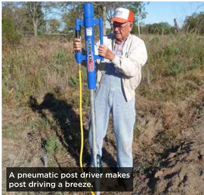
Using a T-post driver in combination with a short driver extension to drive a ground post
