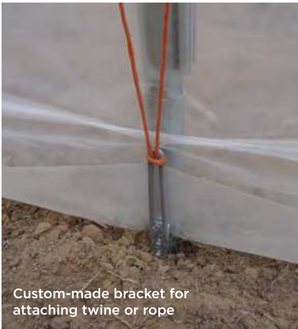
Use of heavyweight baling twine to fasten poly cover to frame. Notice the placement of the rope on either side of the hoop.
