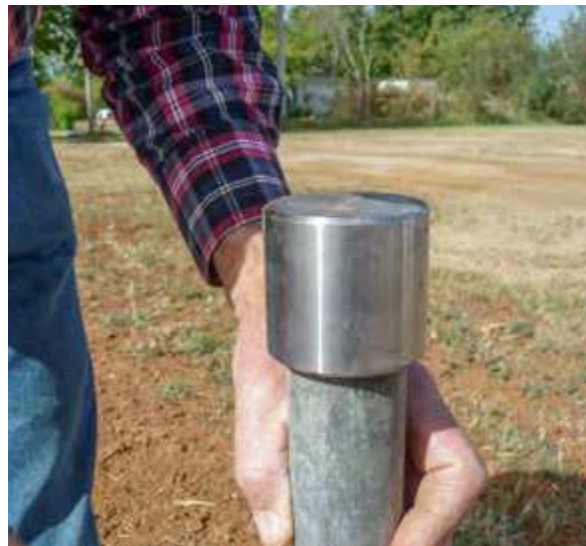
House interior A ground post being installed on the outside of the string line
