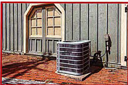
X Inappropriate Prominent unscreened mechanical equipment on the sidewalk
