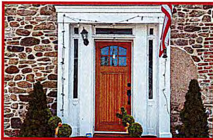
✗ Inappropriate Modern Craftsman style door is not compatible with Greek Revival style entry
