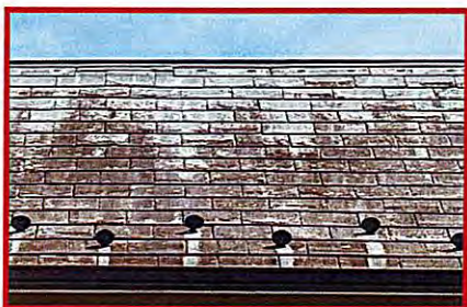
X Inappropriate lack of regular maintenance of slate roofing may cause water infiltration
