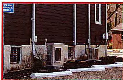
X Inappropriate Visible unscreened mechanical equipment and conduit
