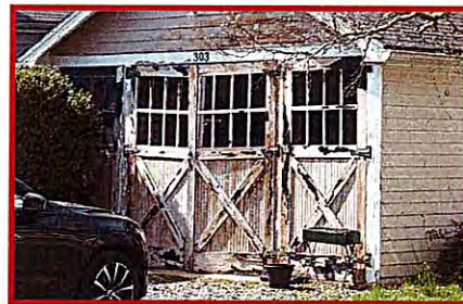
✗ Inappropriate Deteriorated garage doors should be restored to match the original to preserve historic character
