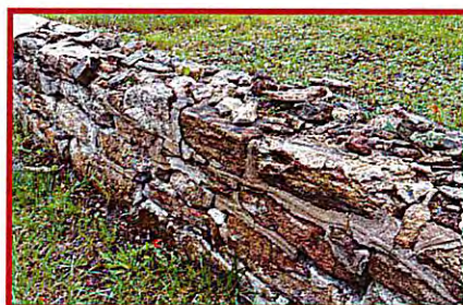
X Inappropriate Stone wall with missing capstone accelerates deterioration and detracts from the site's integrity of design
