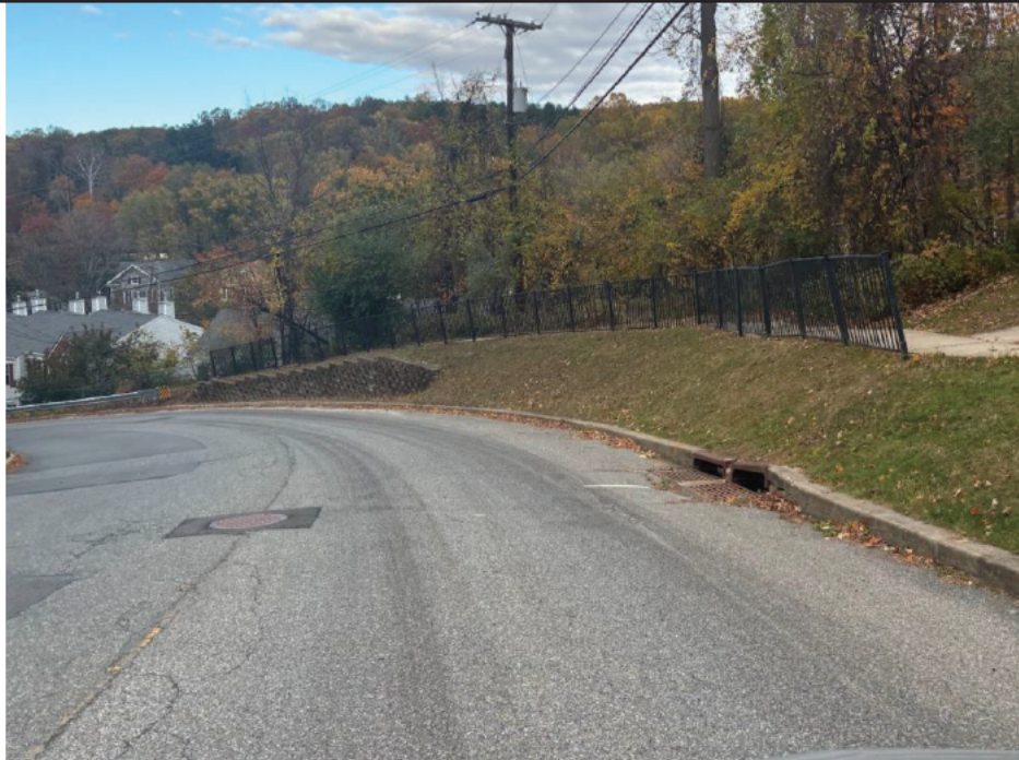
Photo 1: Non-compliant and broken inlets. Fencing to be replaced. Sidewalk repaired as needed.
