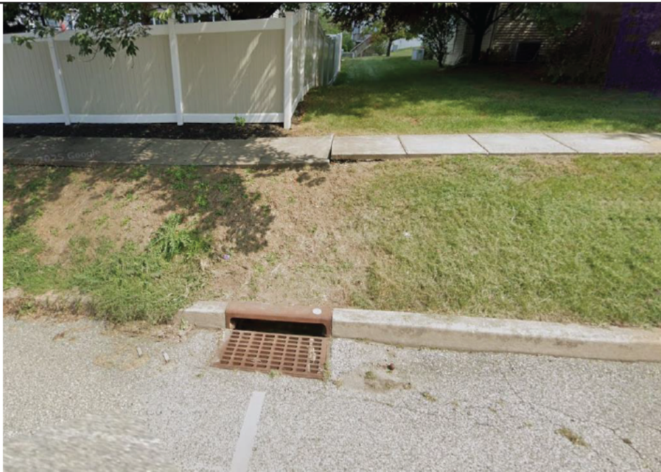
Photo 6: Heaving sidewalk. Non-compliant inlet.
