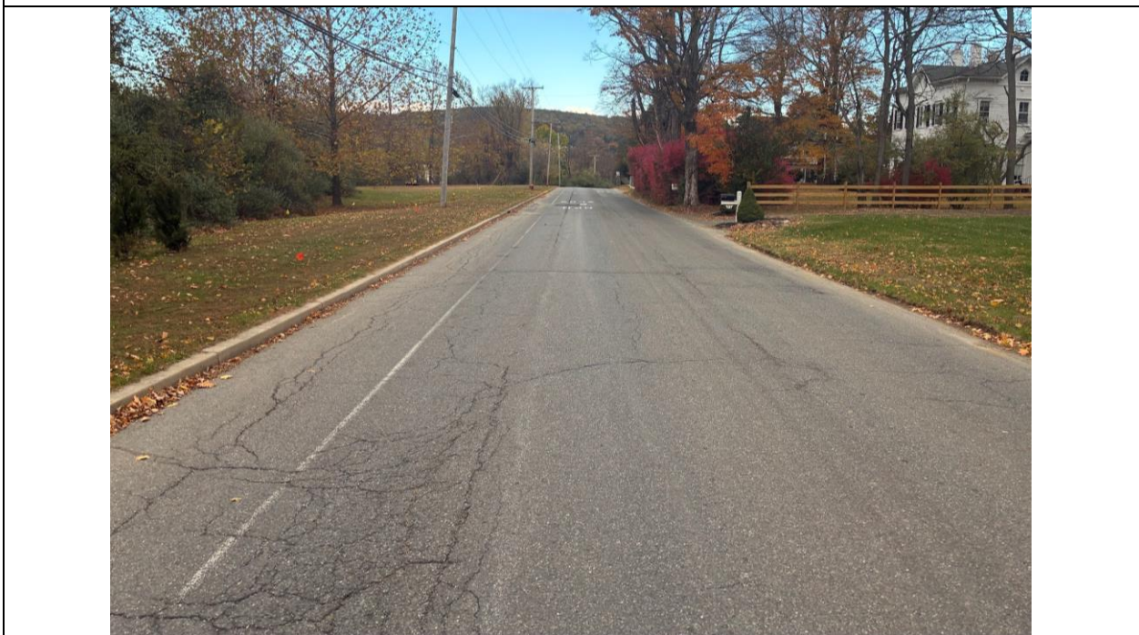
Photo 4: Longitudinal and alligator cracking on roadway. New sidewalk proposed on left side.
