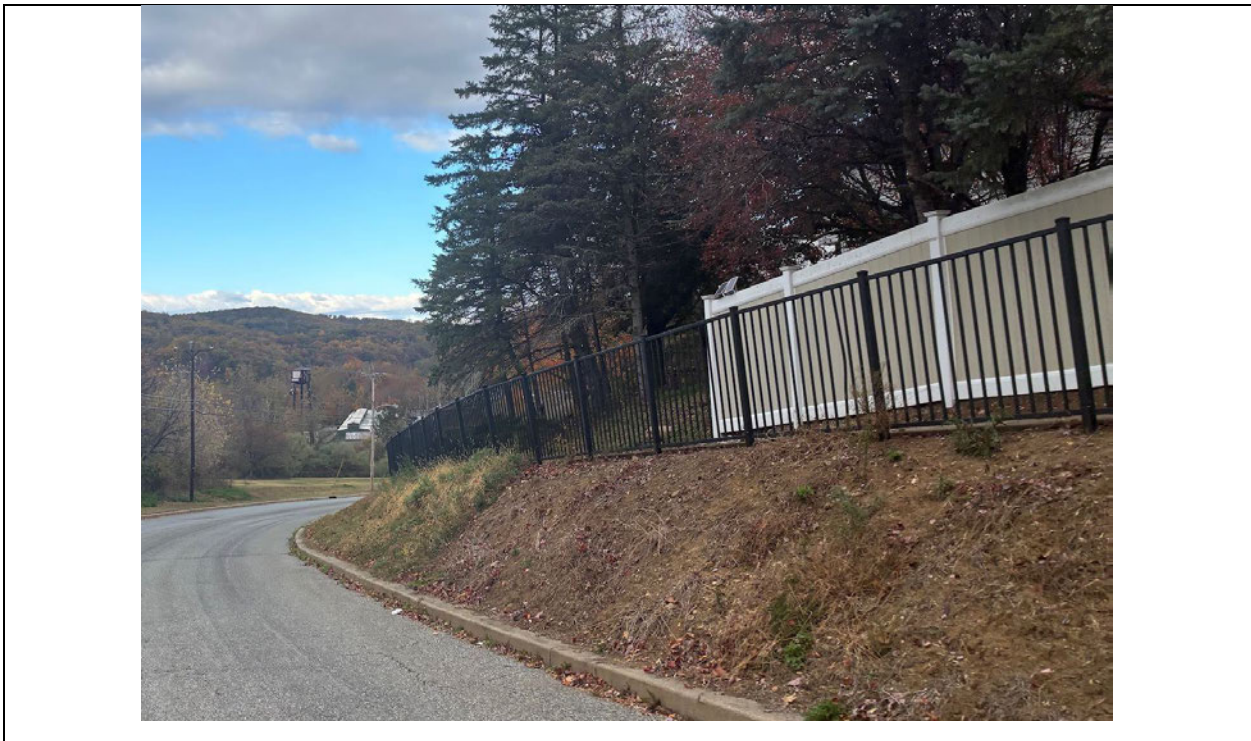
Photo 3: Fencing to be replaced.
