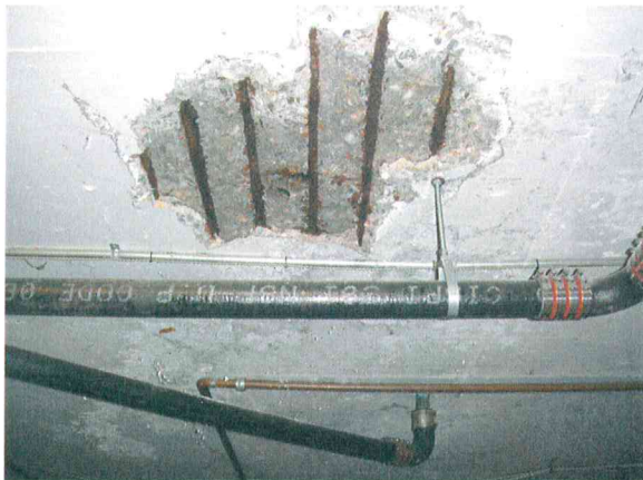
Rusted rebar with large spalled area near patch observed from above
