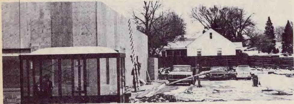
Cold December hasn't dissuaded construction crews working on three different projects in Highland Village. Falling temperatures and a sinking sun have been accompanied by the rising of a new Firestone automobile service center at Ford Parkway and Mount Curve Boulevard (upper left), the Village Mall and its three-level atrium at Ford Parkway and Finn Street (upper right), and a new Kentucky Fried Chicken restaurant at Cleveland and Pinehurst avenues (above).
