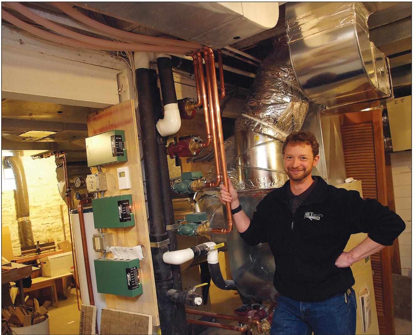
Charlie Dana of Jet Construction & Remodeling shows off the heat pump and exchanger portion of a geothermal system his company recently installed in a Summit Hill home. PHOTO BY BRAD STAUFFER
