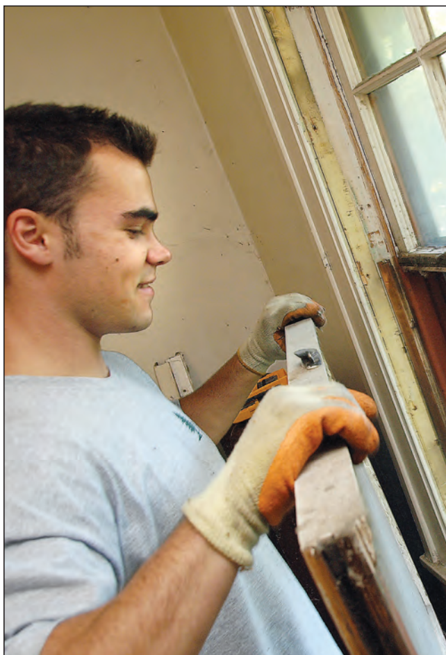
Zach Fredrickson of Nilles Builders repairs a window in a Lexington-Hamline home being rehabbed with the help of the Housing Resource Center. PHOTO BY BRAD STAUFFER
