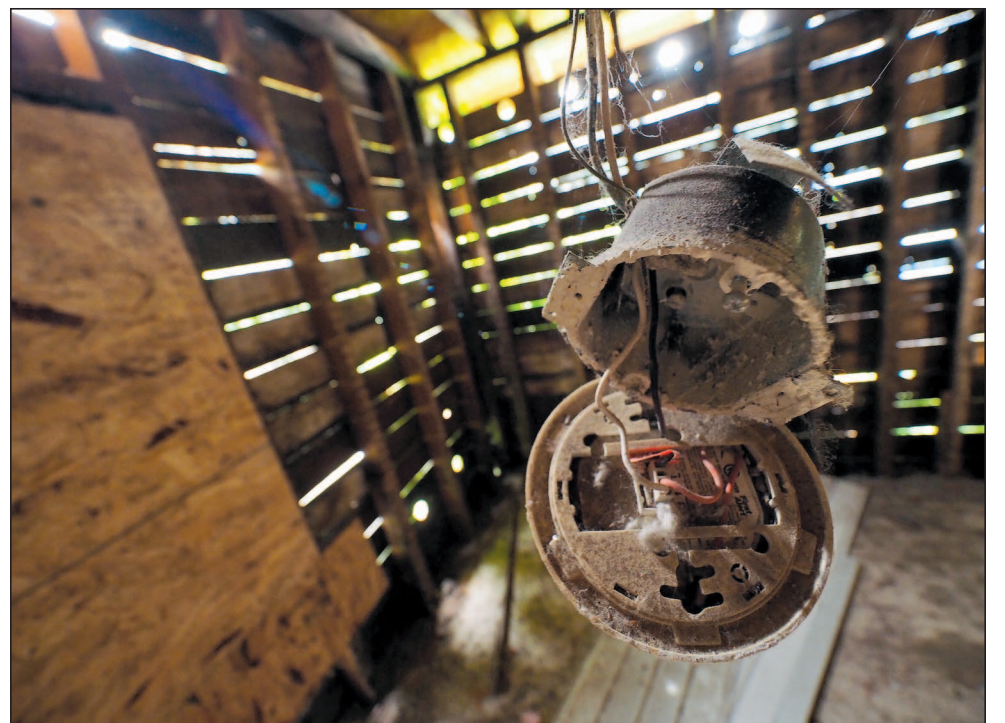
A light socket dangles inside the historic John Lewis House, which has had its siding removed for the time being. PHOTO BY BRAD STAUFFER
