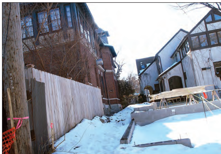
Work on a new garage and two-story addition has halted while the owners of the Portland Avenue home attempt to settle a dispute over the project with the owners of the house at left, Garrison Keillor and Jenny Lind Nilsson.
