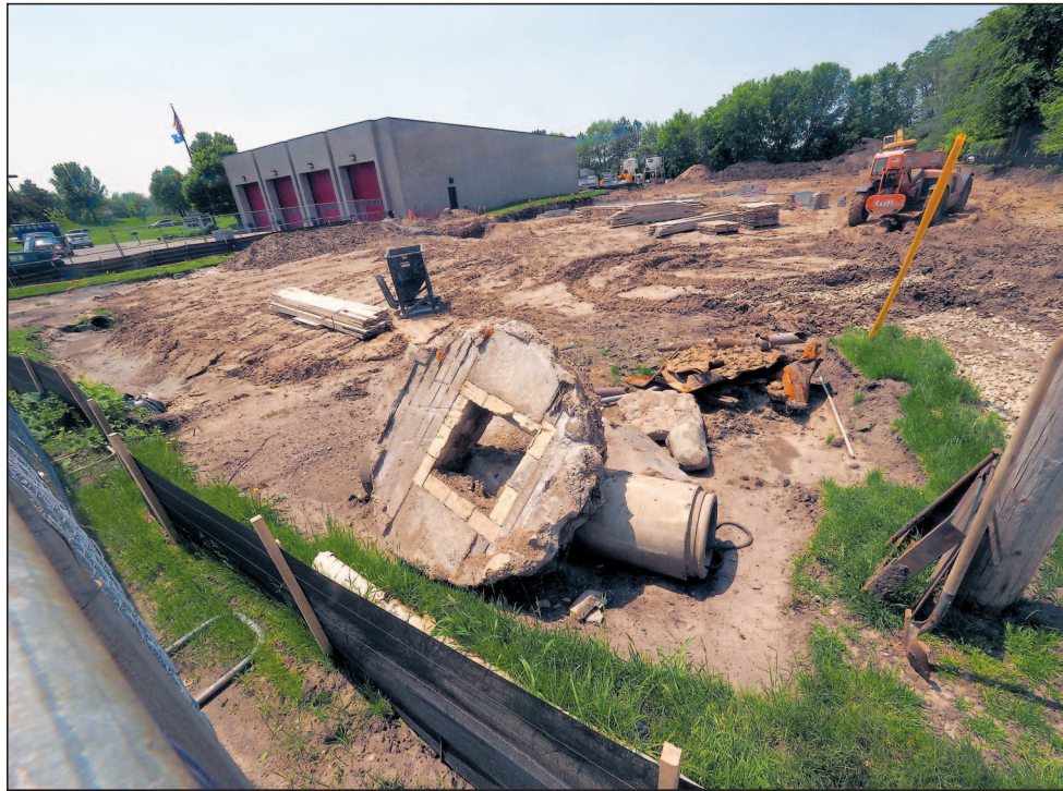
Construction began last month on an $8.1 million project that will nearly double the size of Mendota Heights' only fire station at 2121 Dodd Road. PHOTO BY BRAD STAUFFER
