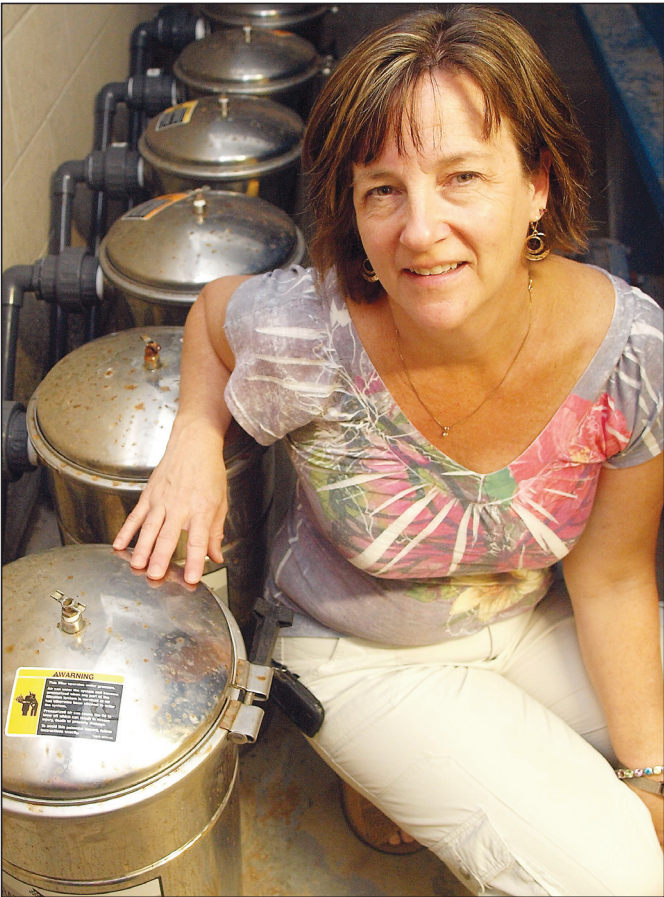
St. Paul aquatics supervisor Lynn Waldorf points out the canisters of sphagnum moss that line the pool filtration room at the Oxford Community Center. PHOTO BY BRAD STAUFFER
