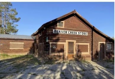
BEAVER CREEK STORE - POTENTIALLY KEEP IF ECONOMICALLY FEASIBLE TO ADDRESS STRUCTURAL ISSUES.
