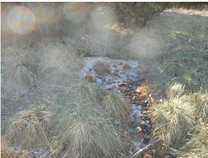
Photograph: # 18. Taken By: Joe Trunko Date Taken: January 13, 2022 Program: WMP-RCRA D Entity: Generally Hauling Sanitary Landfill Permit: 107104 Location: North slope of landfill Description: Leachate outbreak on lower west side of north slope.
