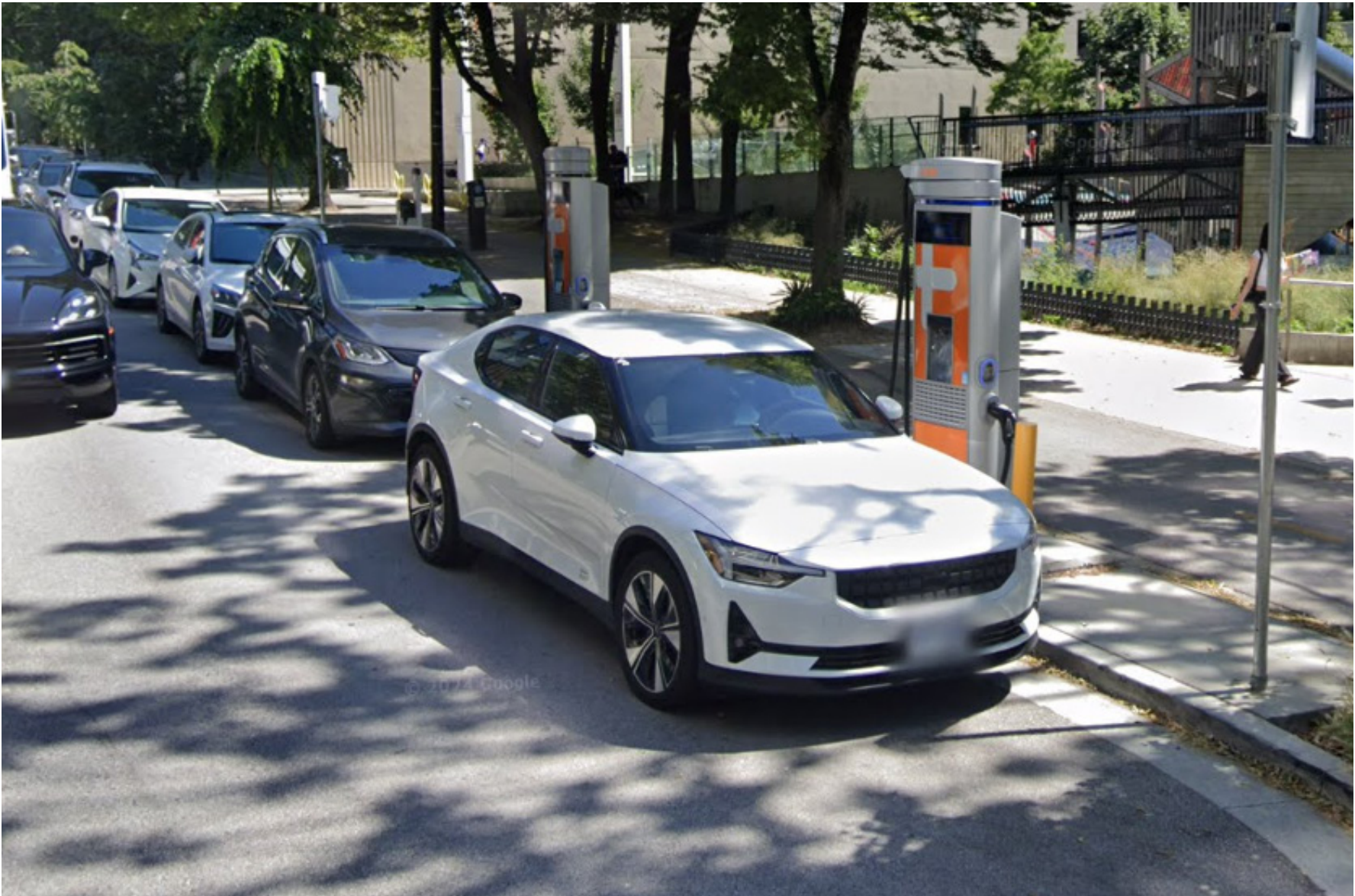
Figure 21: Curbside Charging in Vancouver, BC, Canada; Google Maps Street View
