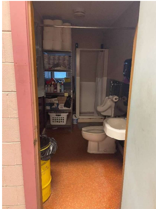
Non-ADA Compliant Bathroom
