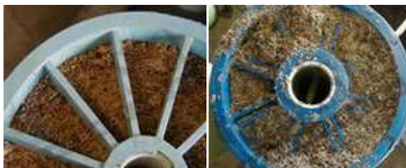
RO elements fouled with resin and sand
