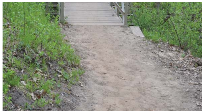
The Rotary Vista Trail was damaged in early 2016 during a January thaw that attracted hikers and resulted in deep footprints in the trail surface. The trail surface was still pockmarked and uneven in late April 2016.
