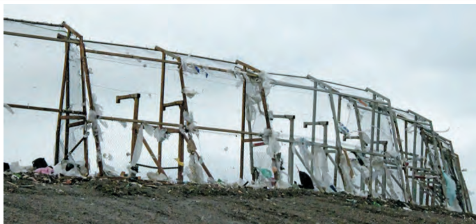
Fences are put in place where crews are working to catch flying debris. Anything that escapes has to be picked up by work crews.
