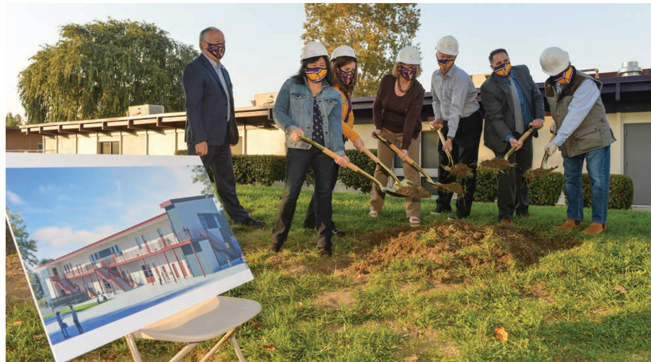
Pleasanton Unified School District Superintendent David Haglund; Board Vice President Jamie Yee; Board Members Valerie Arkin, Joan Laursen and Mark Miller; Amador Principal Joshua Butterfield; and Board President Steve Maher break ground for a new Amador Valley High School building. Both Amador and Foothill high schools celebrated new site developments in events held on Oct. 29. (Photo - Doug Jorgensen)
