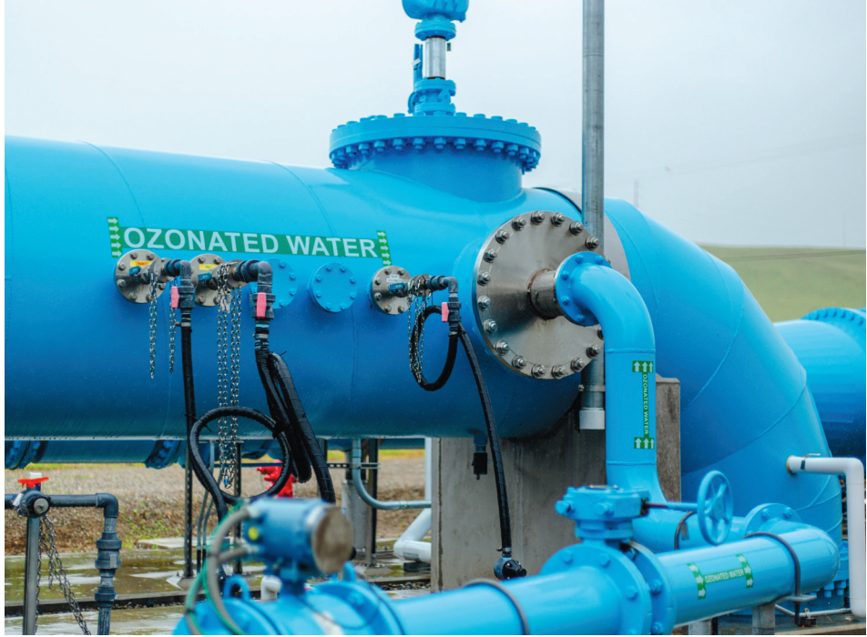
Pictured here is the advanced ozonation infrastructure at the Livermore Patterson Pass Water Treatment Plant. This system is actively used to target and remove seasonal taste and odor compounds from our surface water supply. (Photo courtesy of Zone 7 Water)
