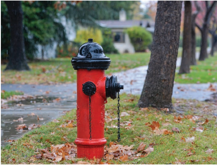
An old fire hydrant is part of the aging infrastructure on Trevarno Road. (Photo - Doug Jorgensen)
