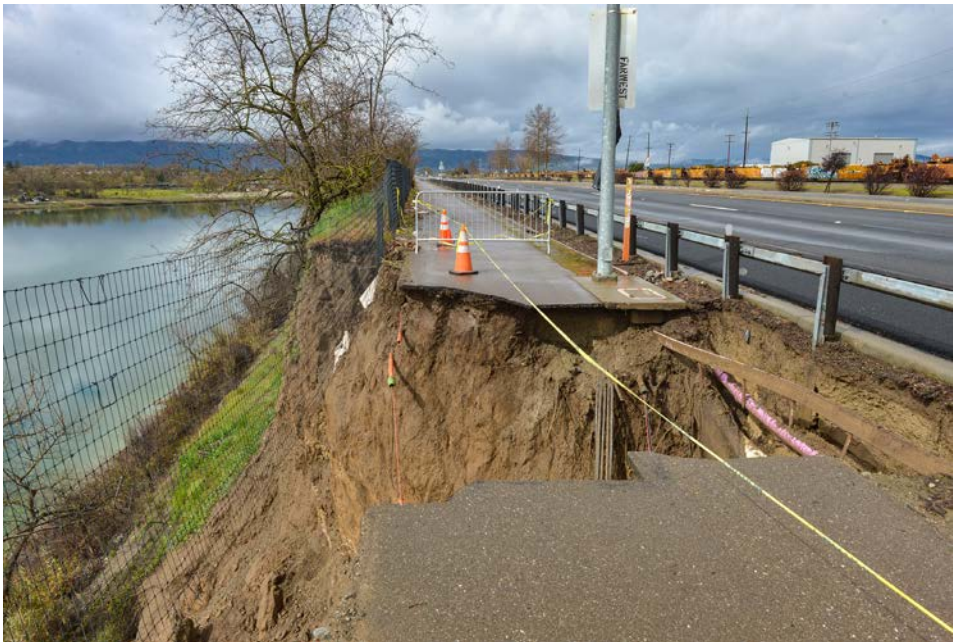
A portion of the path adjacent to Stanley Boulevard in Pleasanton collapsed over the weekend, following another string of atmospheric river storms. The slide resulted in the closure of eastbound vehicular traffic. One lane opened to traffic on Tuesday, March 14. (Photo - Doug Jorgensen)
