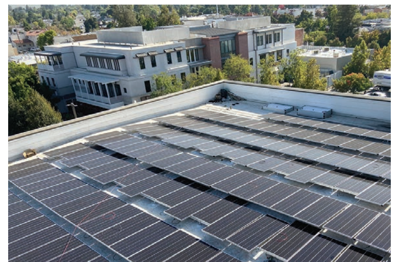
Solar panels placed atop the Bankhead Theater save both energy and money. (Photo - S. Kenison)
