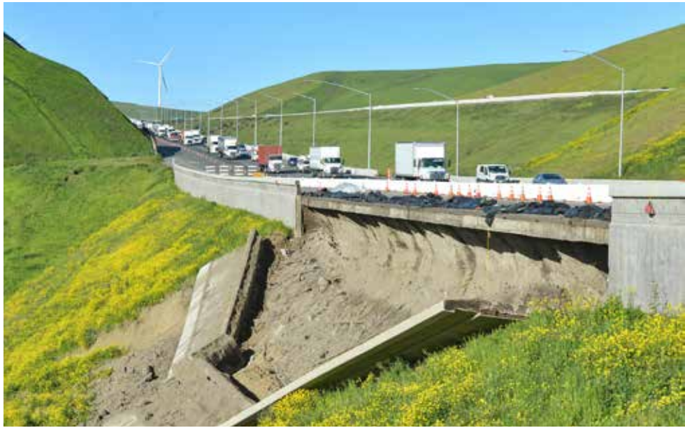
Lane closures on Eastbound 580 stopped traffic for hours during storm weather in March. Caltrans worked to shore up a retaining wall that slid during the series of storms.
