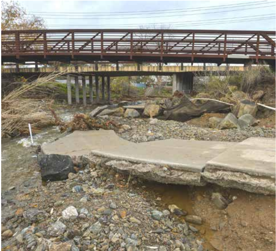
The Arroyo Bike Path in Livermore at Concannon Boulevard experienced significant damage during the New Year's storm.
