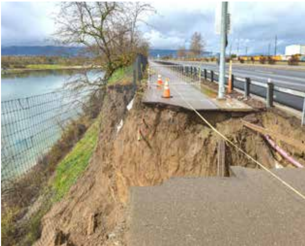
A portion of the path adjacent to Stanley Boulevard in Pleasanton collapsed over the weekend, following another string of atmospheric river storms. The slide resulted in the closure of eastbound vehicular traffic.
