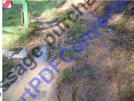
Hunters violating gated road-closures is another common problem.
