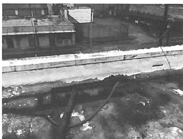
Exposed wiring through roof
