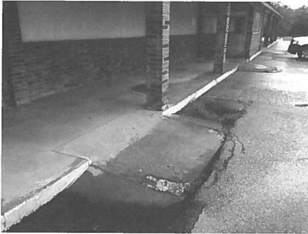
Ponding at inadequate accessible locations
