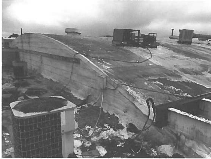
Existing roof top mechanical equipment
