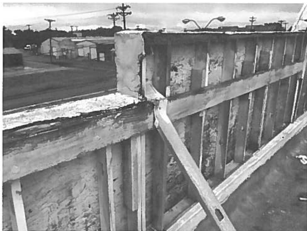
Inappropriate construction at parapet
