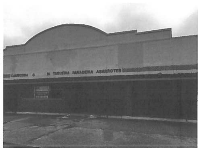
Top parapet should be removed
