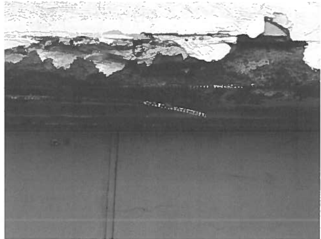
Damage at head of door
