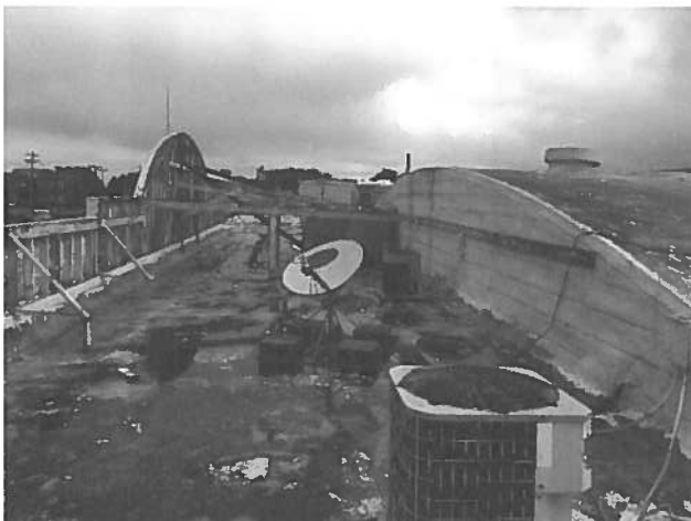
Ponding on flat roof area
