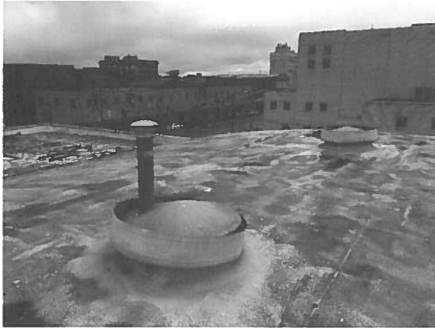
Vent covered not properly sealed
