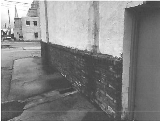
Roof runoff damaging wall surface
