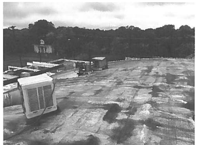
Foamed material causes ponding
