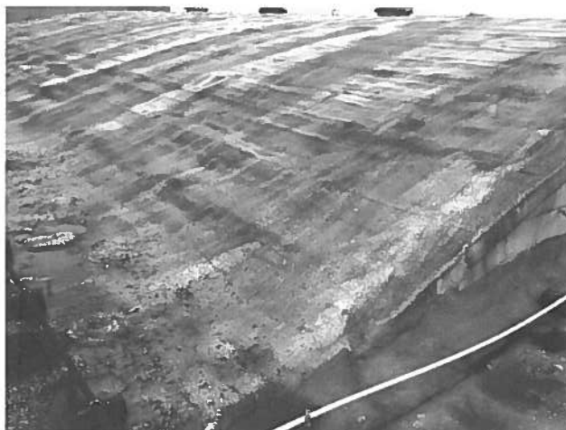
Open blisters on roof
