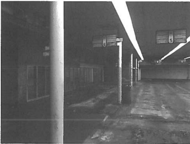
Unprotected steel tubes
