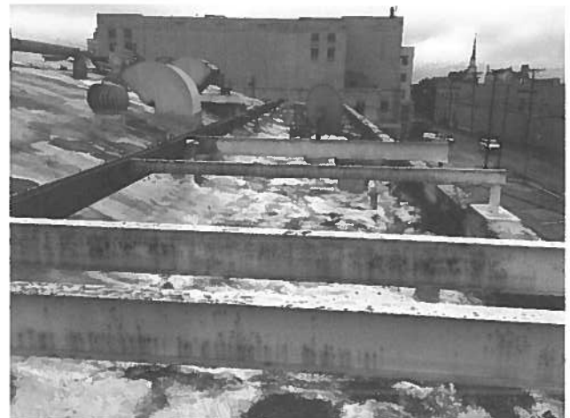
Exposed steel on low roof sides
