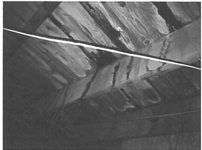
Water damage under roof
