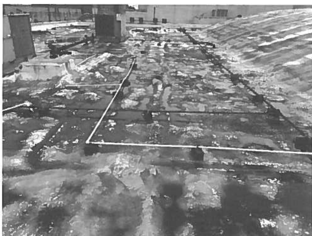
Condensate drains not connected
