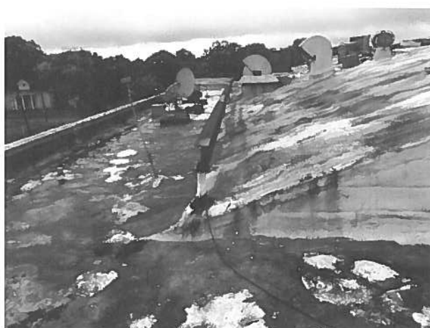
Numerous openings in surface
