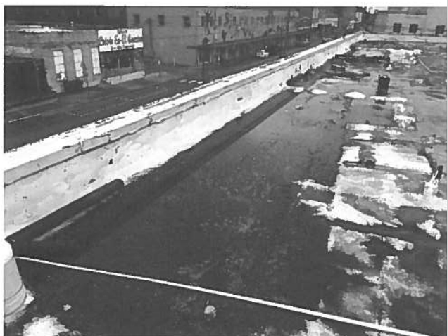
Massive ponding along north side
