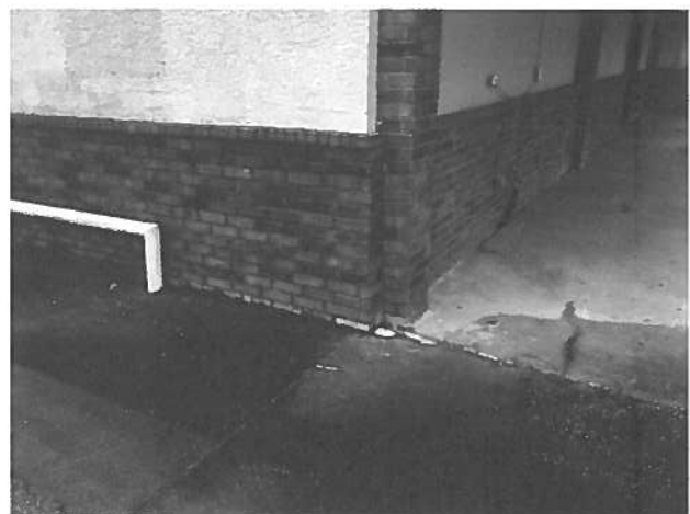
Ponding along north elevation
