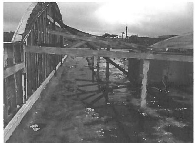
Poor bracing at parapet
