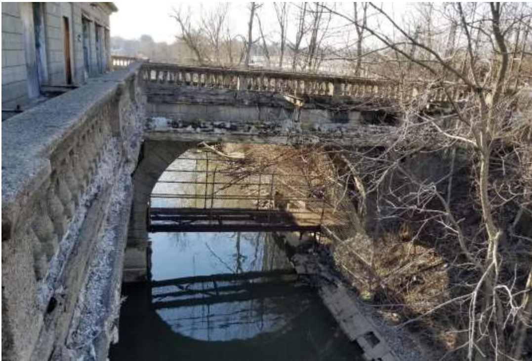
Figure 6. View of the concrete bridge connecting the building to the adjoining causeway. Note the steel walkway below the main span.
