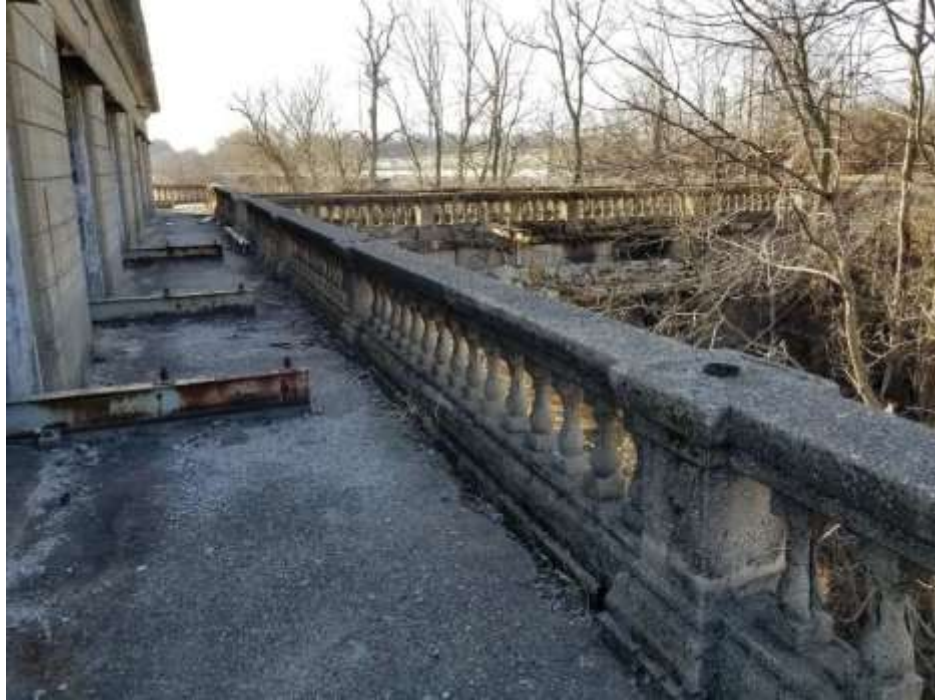
Figure 8. View of the balcony running along the upper level of the building. The steel I-beams running along the deck support a large water pipe below the balcony and represent a later addition.
