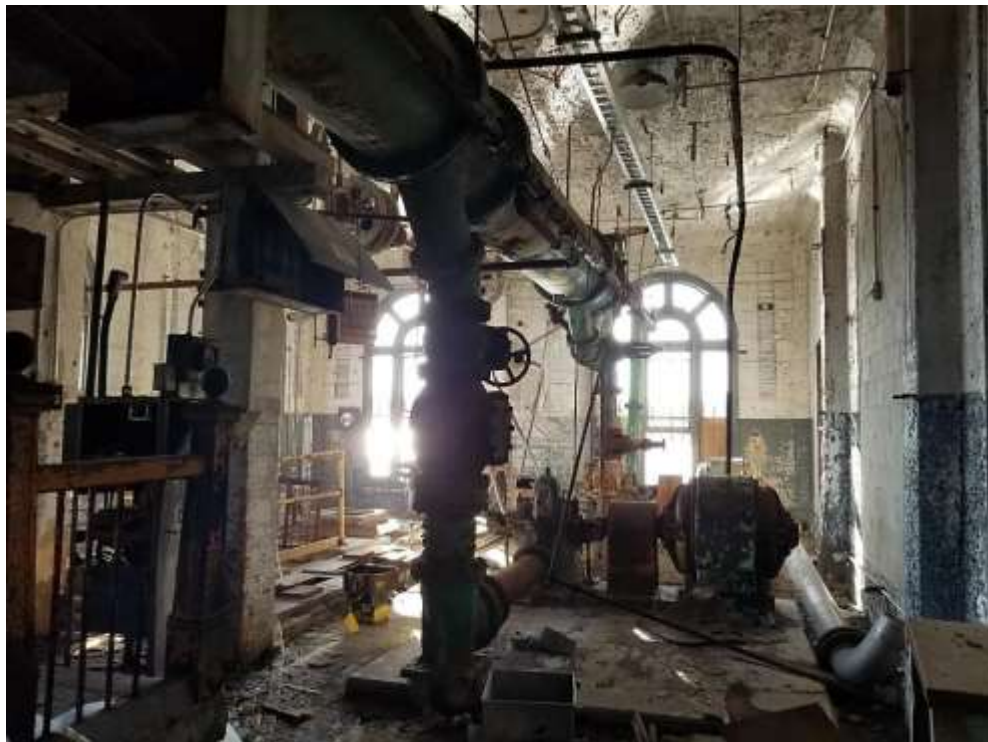
Figure 14. Views of the southern end of the pump room on the Landing Level of the building.
