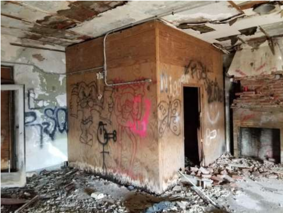
Figure 12. Views of the northern room in the Balcony Level. This room, which originally served as the “club room”, also has a fireplace and multiple sets of exterior doors leading out onto the balcony. A small chamber has been framed out in the corner of the original room.
