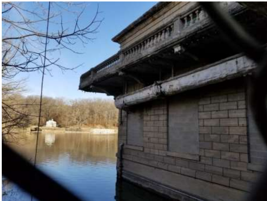
Figure 9. View of the west elevation of the lower, or Landing Level, in which the pump room is located. The window openings on this elevation have been enclosed with concrete block. Note the large water pipe running below the balcony.
