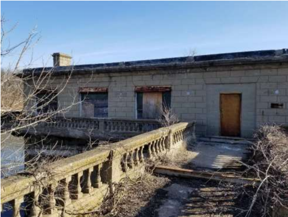
Figure 7. Views of the west elevation of the Balcony Level, taken from the bridge by which it is accessed.
