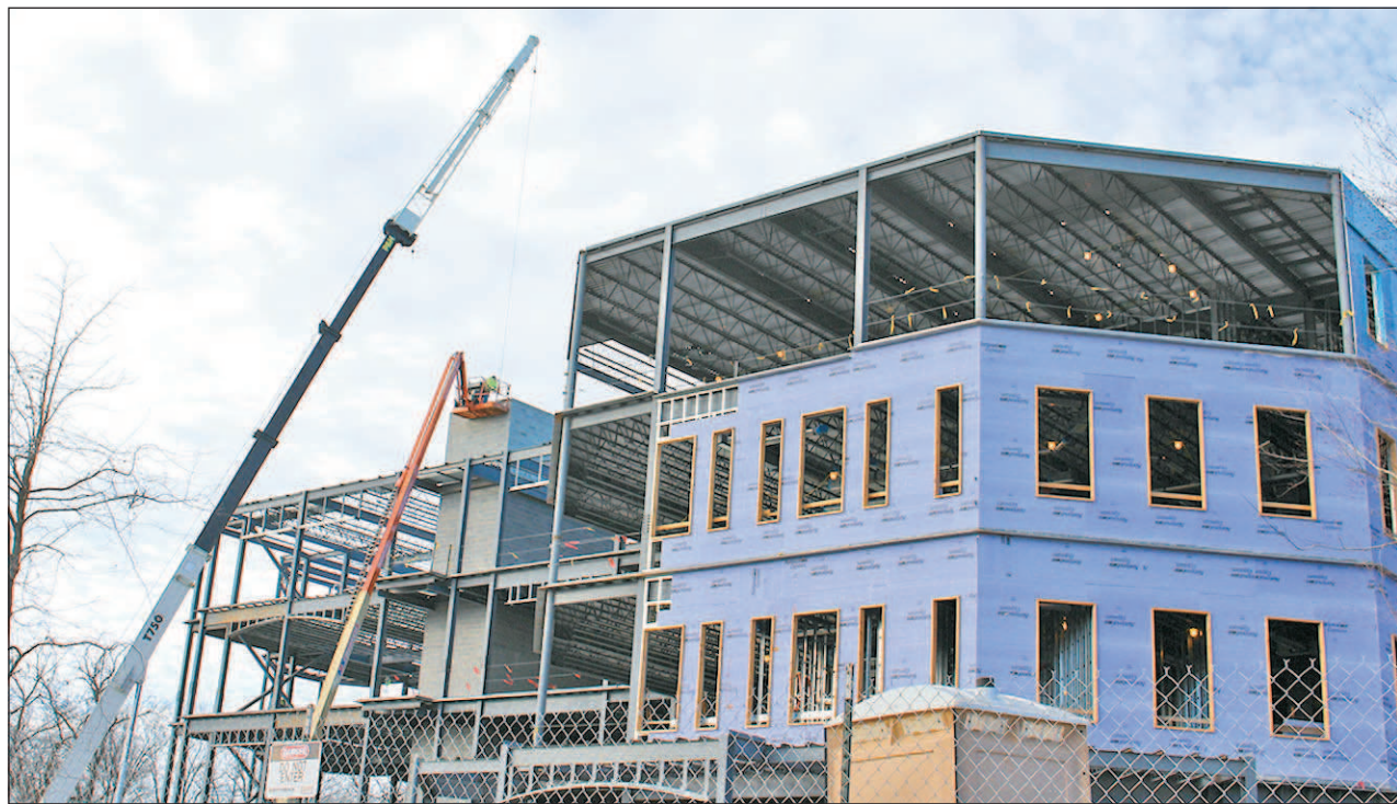
Progress has been steady at the site of Tusculum College's new Ronald H. and Verna June Meen Center for Science and Math, under construction since May 2015. The four-story, 100,000 square-foot facility is expected to be completed in September 2016.
