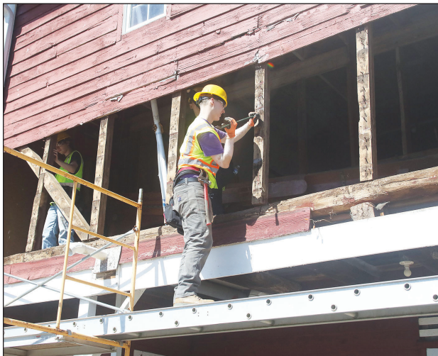
Linkin Heagy from the Adams County Technical Institute removes the old nails from the beams in the Ditzler Barn in Biglerville. It is the home of the National Apple Museum. (Darryl Wheeler/Gettysburg Times)
