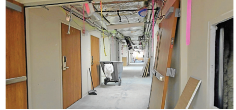
Work continues in the behavioral health unit's hallway, which has wires, hoses and pipes visible during construction.
