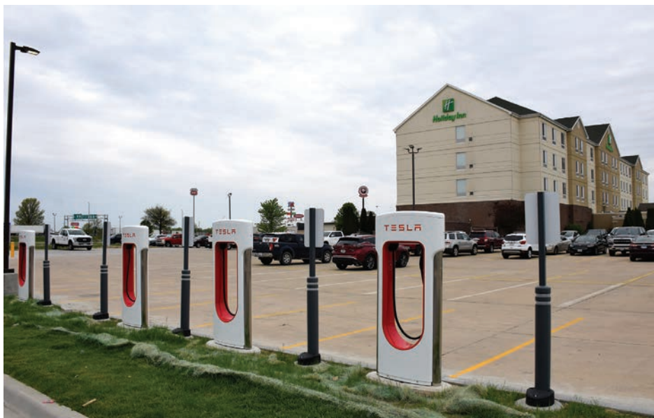
In the parking lot of the Holiday Inn in Effingham, there are several Tesla Superchargers so drivers can charge their electric vehicles. Nick Taylor photo
