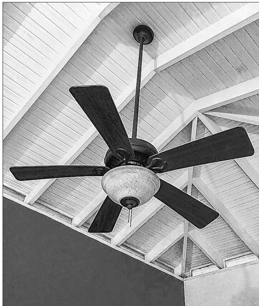
Reversing ceiling fans in winter can help redirect warm air from the ceiling into living spaces below.
