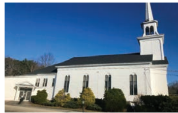
Four pairs of the sanctuary windows as seen on the north face of building.
