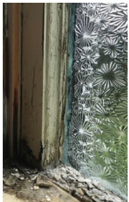
Detail of sash deterioration.
