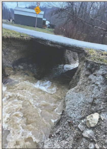
SUBMITTED PHOTO The washed-out culvert at Barbeque Road and Barbeque Spur is pictured.
