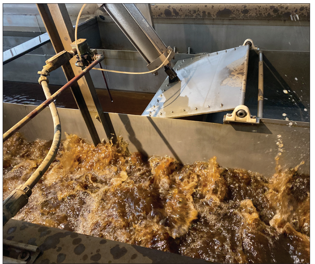
Partially treated water bubbles while being flushed by a filter at the city's water treatment plant. The organic matter is removed from the water then sent to a backwash tank for future treatment.
