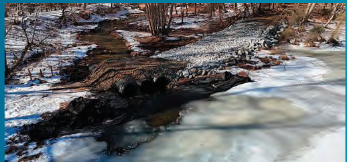
The Cypress Branch Dam Removal Project was completed in April of 2025 reopening over 35 miles for herring, hickory shad, and more.
