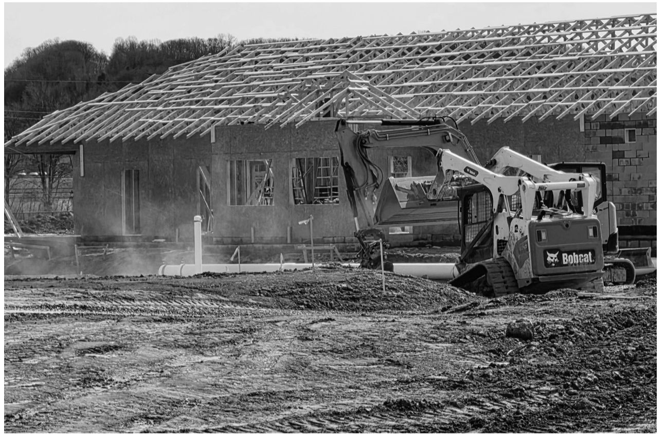
Staff photo by Charles Owens The unseasonably warm weather the region experienced earlier this month has allowed construction crews to make significant progress on Princeton's new wave pool and bath house project with both the walls and roofing on the bath house now going iup.
