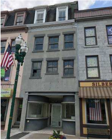
Exterior view – inside is gutted with water damage.
