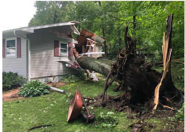
Damage to Residence
