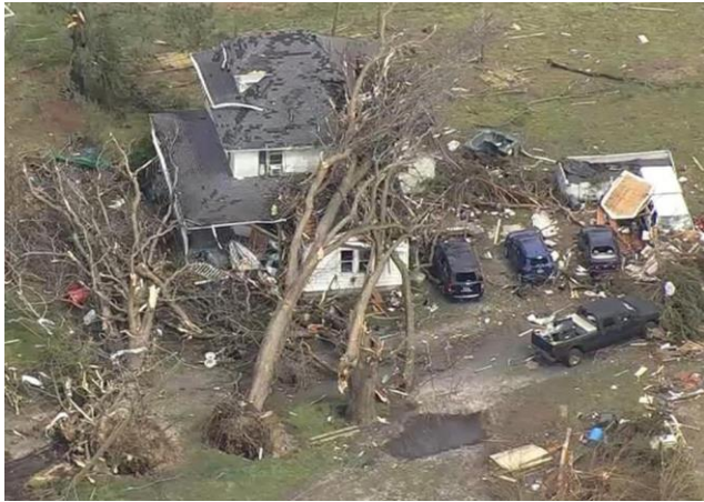
Damage to Residence
