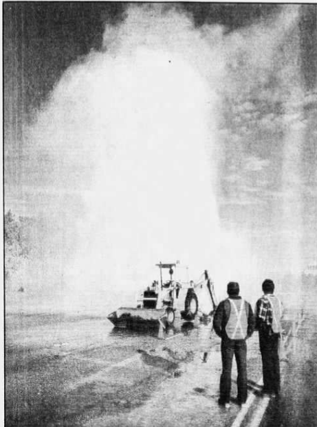
Downtown gusher — Tucson water department employees George Clark and Luis Lopez watch as a broken 16-inch water main sends a jet of water 100 feet into the air. The burst line left some downtown residents without water for 30 minutes or more. Steve Jilb
