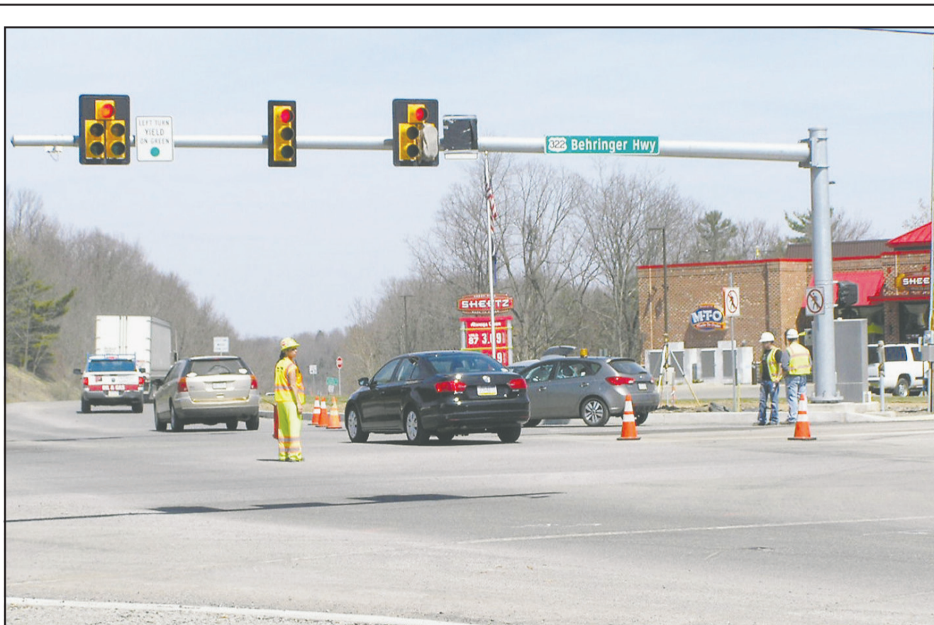
Motorists carefully negotiate the intersection of route 322/119 near the new Sheetz store south of DuBois. Flaggers from HRI Inc. help direct drivers as paving and construction work continues on the road near the light. The light has been put on "flash" and drivers are urged to use caution when negotiating the area and to have patience when traffic backlogs occur. (Photo by Kimberly Finnigan)
