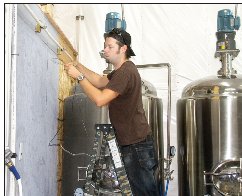
John Boczar, head distiller at Grand Teton Vodka, wires fermenters for automation at the plant.
