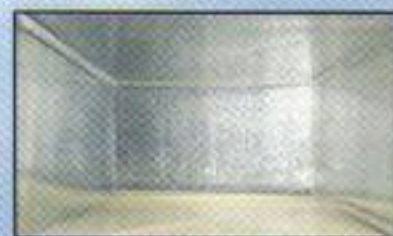
Air duct after cleaning
