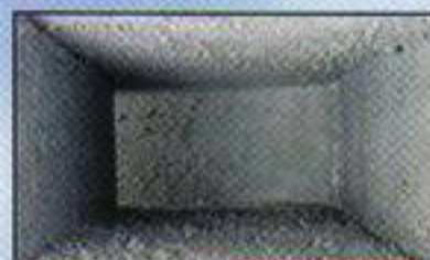
Air duct prior to cleaning
