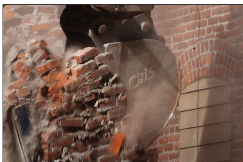
TUMBLING DOWN: Bricks are torn from the side of 200 Main St. Wednesday during the building's demolition.
