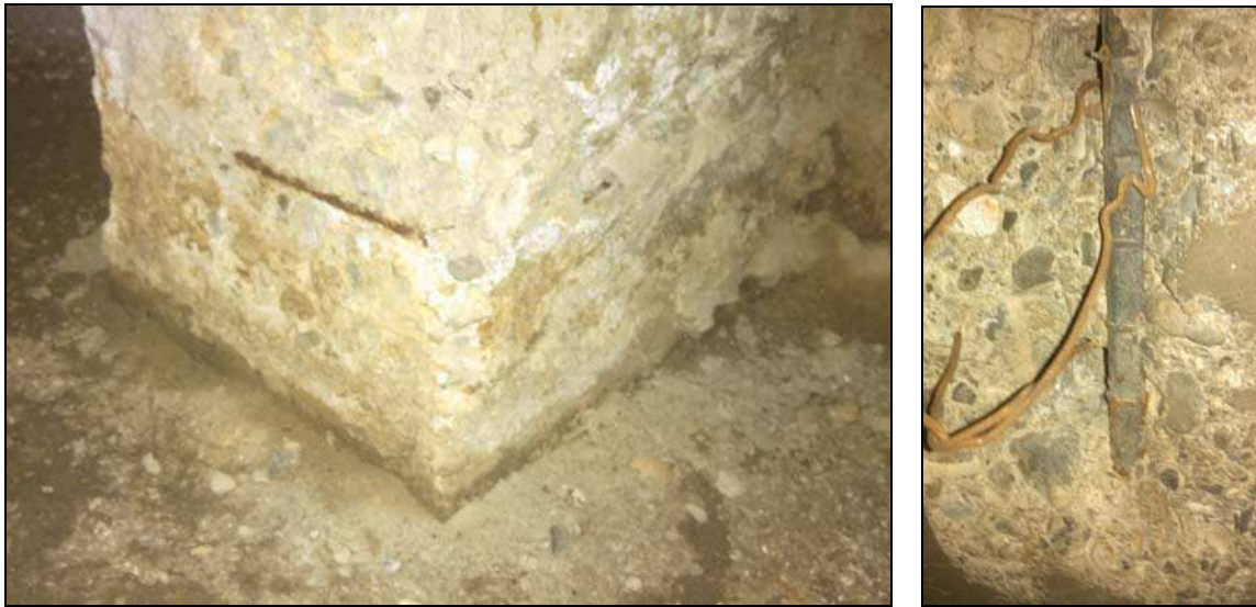
Figure 5: The concrete is deteriorated at the column bases in the sub-basement. In several locations, the concrete is spalling away and the reinforcement is exposed, leaving it susceptible to further corrosion and damage.
