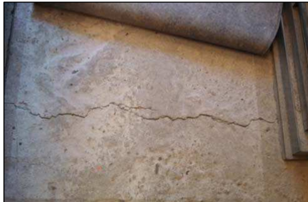
Figure 4: Cracking in the concrete roof slab.
