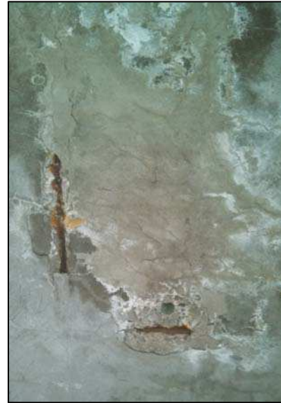
Figure 3: Spalling and exposed reinforcement on underside of slab at the main entry.
