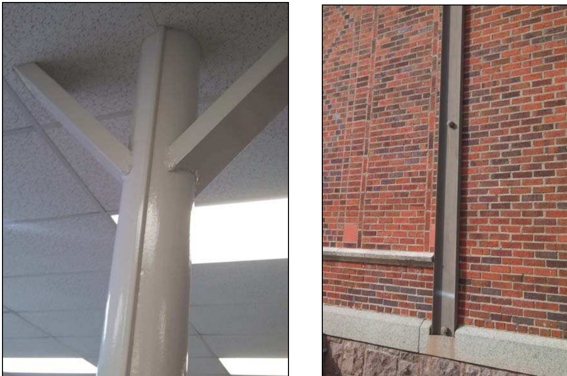
Figure 2: Post-construction retrofits. Steel columns and knee braces found in the classrooms in the original building portion are shown left and steel channels added to the exterior unreinforced masonry walls are shown right.
