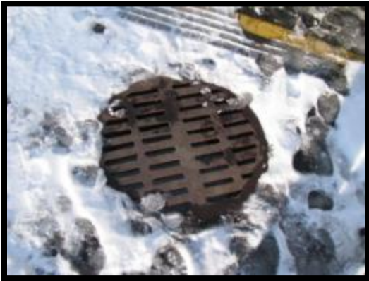
Parking Lot Storm Drain
