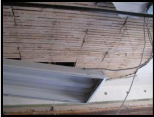
Ceiling Damage in 2 nd Floor of Story Mansion
