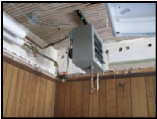
Temporary Heating 2 nd Floor of Story Mansion
