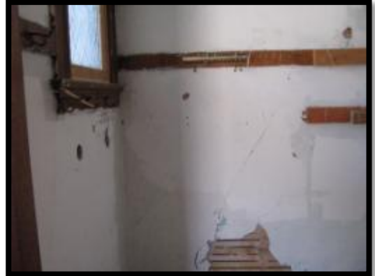
Wall Damage in 2 nd Floor of Story Mansion
