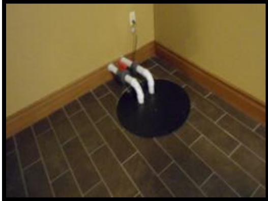
Basement Sump Pump
